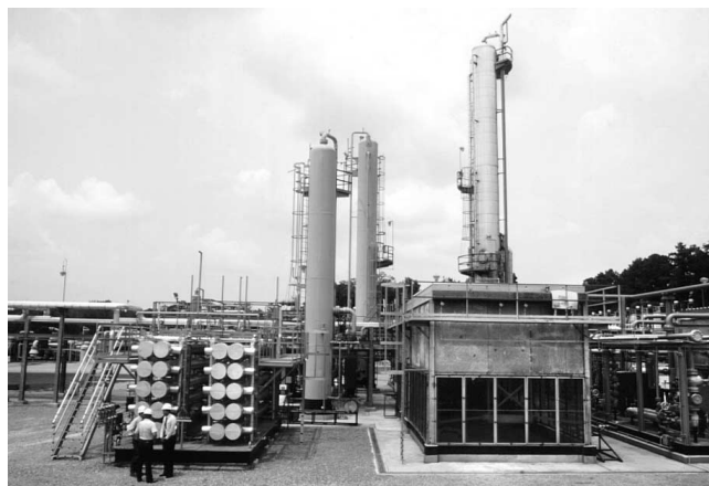
Figure 6. The skid in the lower left replaced all the units to the right (Dortmundt, 25)
