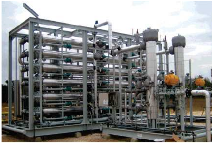
Figure 5. A CO 2 membrane separation plant. This is a 9 million scfd membrane plant designed to reduce a 6% CO 2 gas to 2%. (Baker, 2113)
